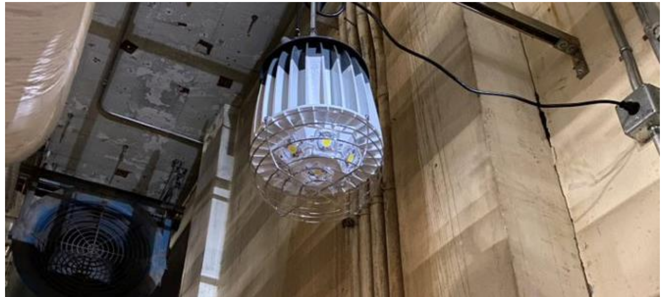
New outdoor fixtures (Boylan Well)/ LED light fixtures (MER)
